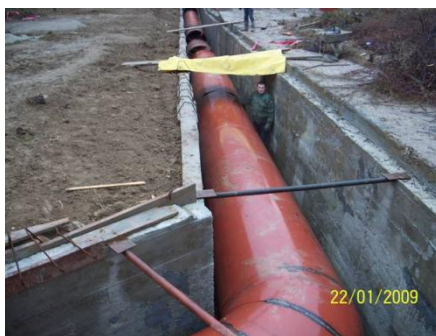
FIG. 8. New ventilation pipeline.
